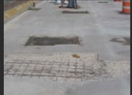
Typical Patch Area
