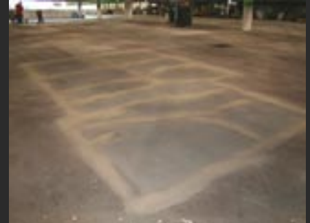
Crack Detail Using EM-100N
