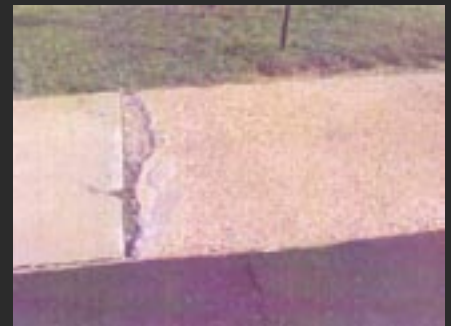
Condition of spalled concrete before SC-111 System
