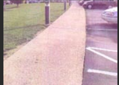
Condition of spalled concrete before SC-111 System
